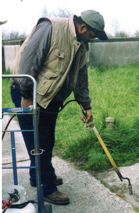
Torches work on weeds in cracks or gravel
